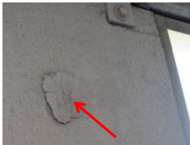
Figure 1: Failing Concrete Patch
