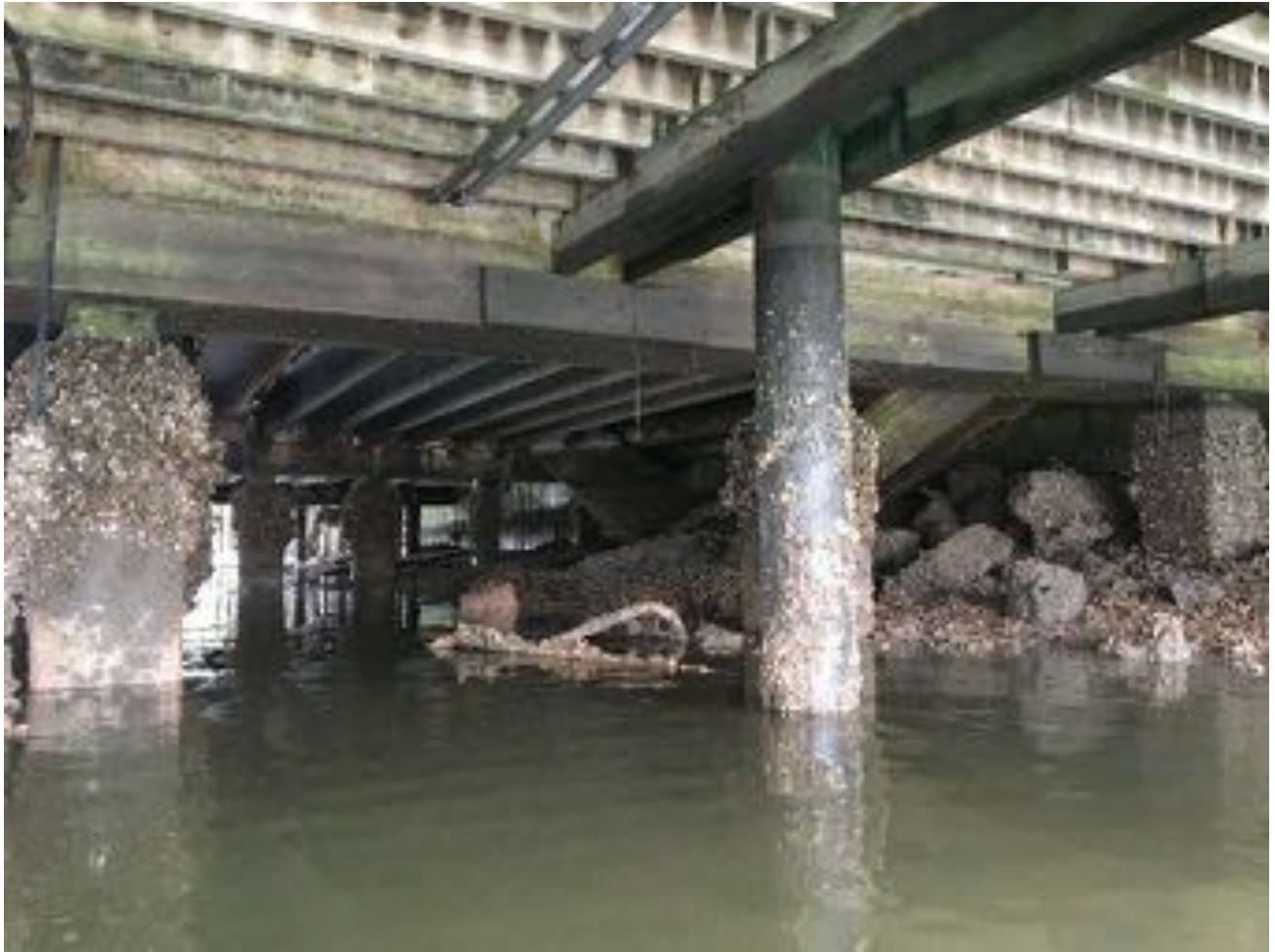
1.05~ Southeast portion of substructure. Timber piles and underside of boardwalk decking in the foreground. Reinforced concrete piles with marine growth in the background. Failed reinforced concrete lower double tee (1962) on righthand side of picture.
