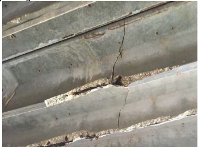
1.23~ Lower double tee with full section crack, missing portions of stem, and deflection.
