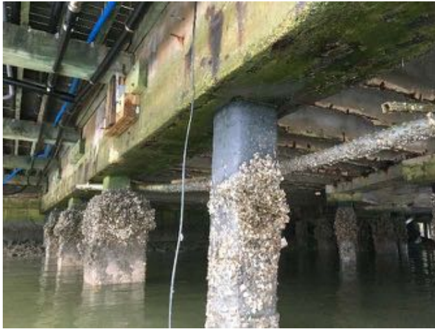
1.32~Northeast area of substructure looking east Lower double tees missing sections of the stem at points of bearing and along the spans; Octagonal area beams in fair condition with some patching; beam in picture foreground has cracking and spalling along bottom; piles with marine growth.
