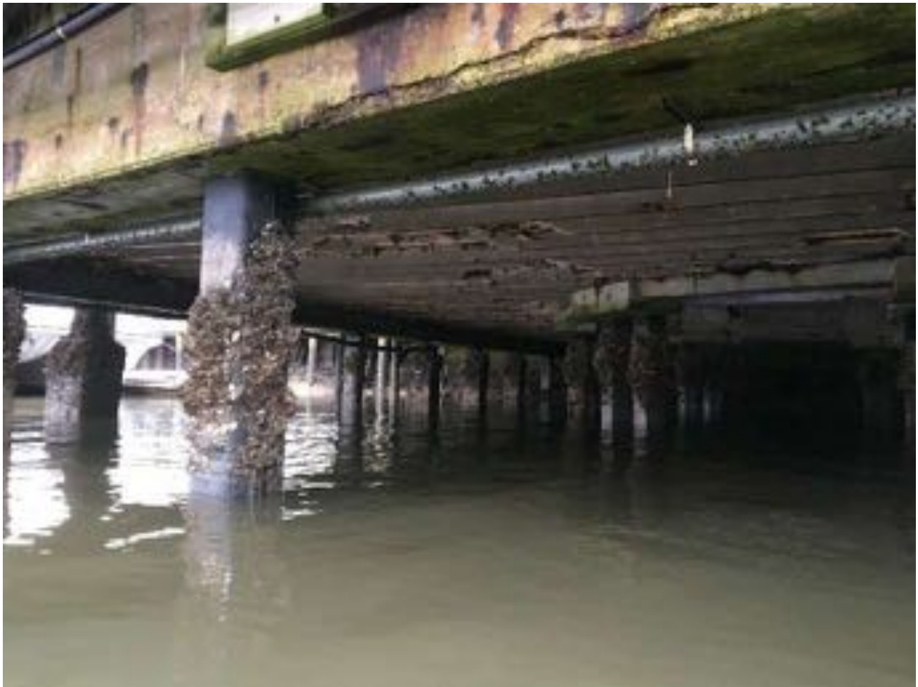
1.14~ West side of substructure looking northeast. Lower double tees with missing sections of the stem at the points of bearing and along the span; concrete beams with missing / spalled concrete and horizontal cracking; piles with some repairs and marine growth.
