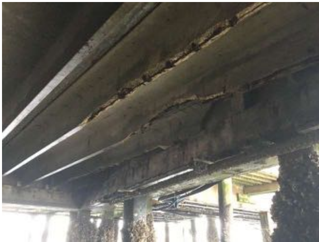
1.26~Southwestern corner of substructure; Lower double tees with missing sections of the stem along the span; concrete beam with horizontal cracking entire length of beam and missing bottom section at pile, righthand side of picture; piles with marine growth.
