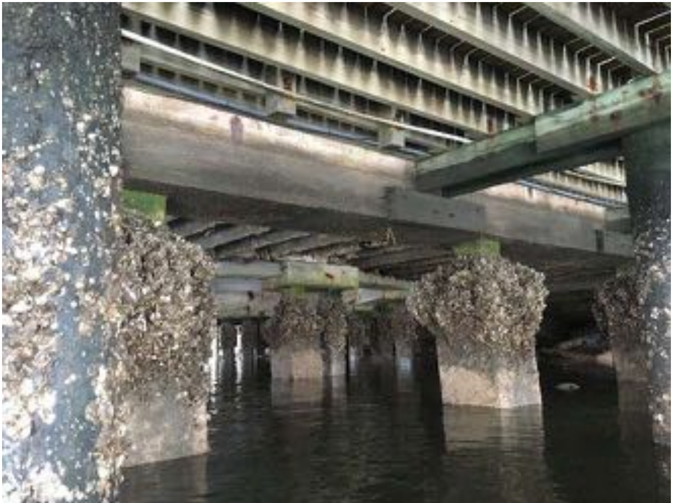
1.09~ South-central portion of substructure looking northeast. Lower double tees with missing portions of their stems. Concrete beams without visible defects. Piles with marine growth.
