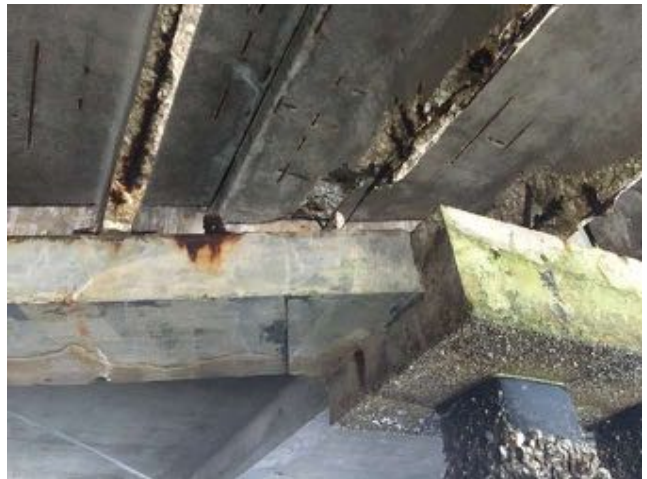
1.21~Lower double tees missing stems. Top of one Lower double tee has deflected. Concrete beams with patching.
