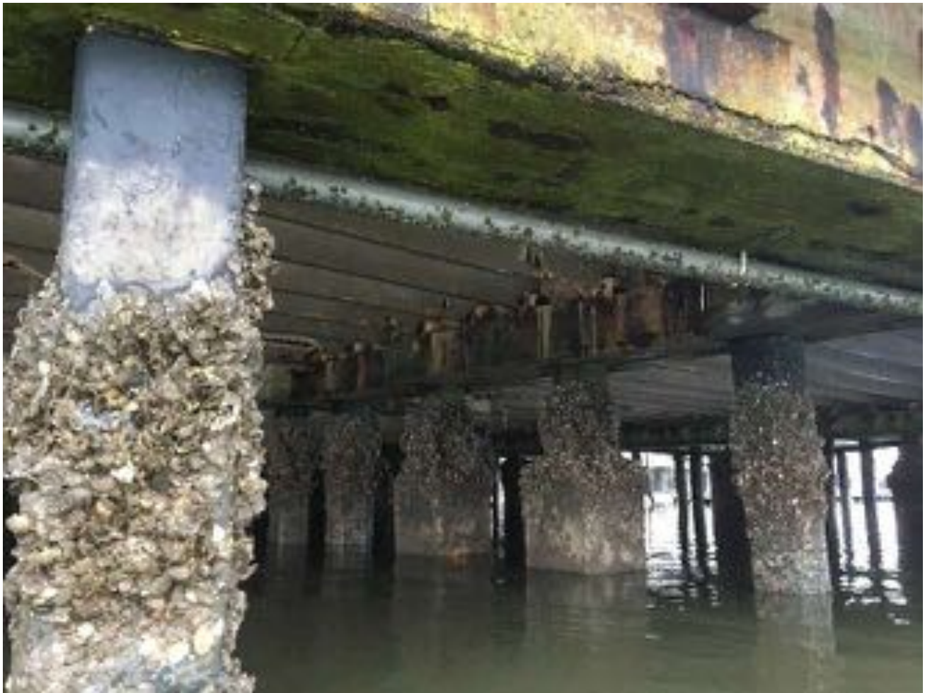
1.16~Lower double tees with missing sections of the stem at the points of bearing and along the span; concrete beams with horizontal cracking; piles with some repairs and marine growth.
