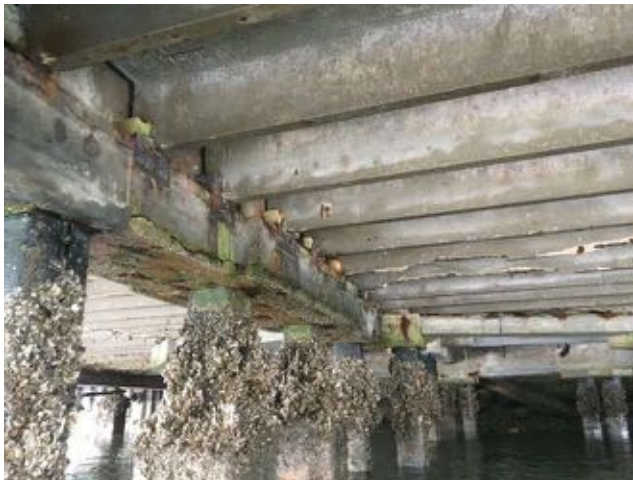
1.24~ Lower double tees with missing sections of the stem along the span; concrete beams with horizontal cracking; piles with marine growth.
