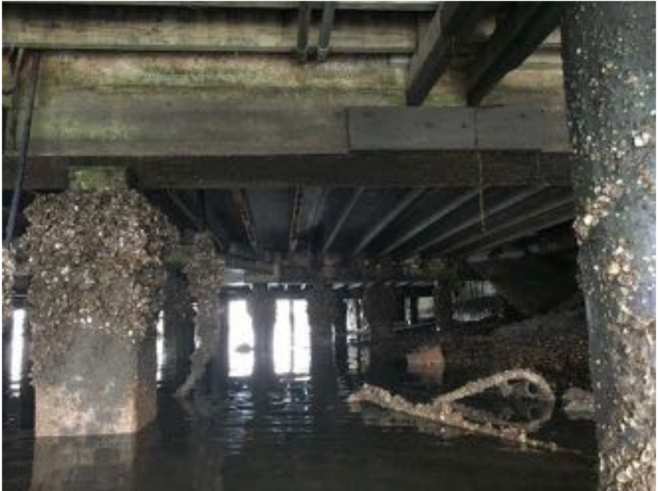
1.06~ Southeast portion of substructure. Timber piles and underside of boardwalk decking in the foreground. Reinforced concrete piles with marine growth in the background. Failed reinforced concrete lower double tee (1962) on righthand side of picture. Other lower double tees missing the bottom of their stems.
