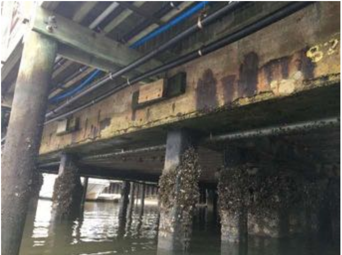
1.13~ West side of substructure looking northeast. Concrete beams with missing / spalled concrete and horizontal cracking; piles with some repairs and marine growth.
