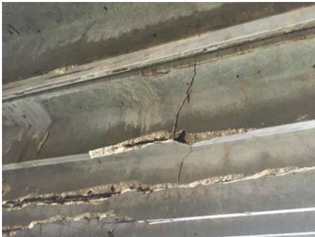
1.22~Lower double tee with full section crack, missing portions of stem, and deflection.
