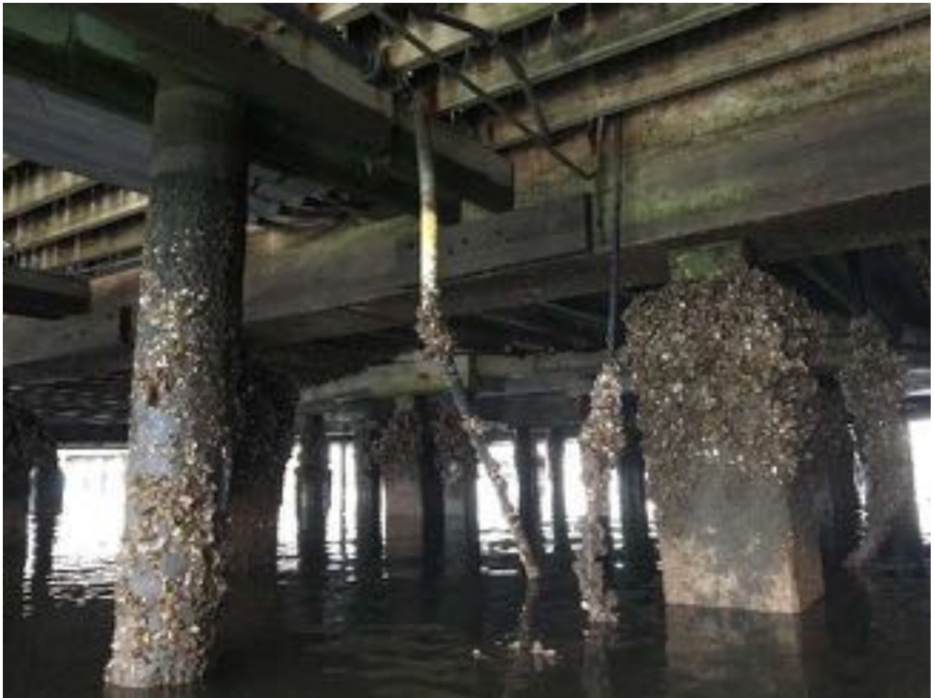
1.07~Southeast portion of substructure looking northwest. Concrete beams without visible defects. Piles with marine growth.
