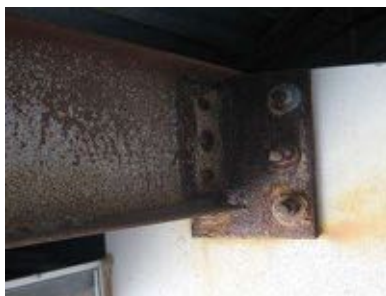
Figure 4: Structural Steel Corrosion and Scaling
