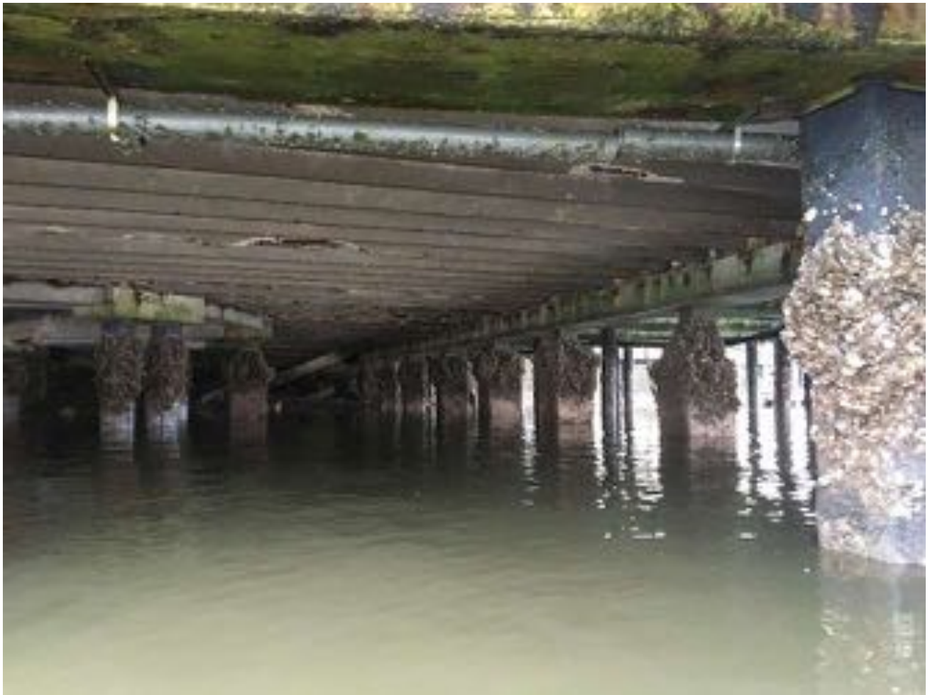
1.11~ Western portion of substructure near south side looking east. Lower double tees with missing portions of their stems. One of the lower double tees has failed and dropped into the river in the background of the picture. Concrete beams with horizontal cracking in the bottom face. Piles with marine growth.
