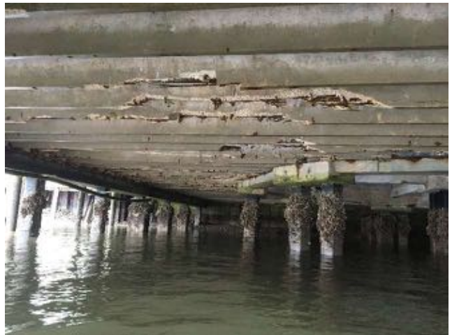
1.29~Northern portion of substructure; Lower double tees with missing sections of the stem along the span; Octagonal area beams in good condition; piles with marine growth.
