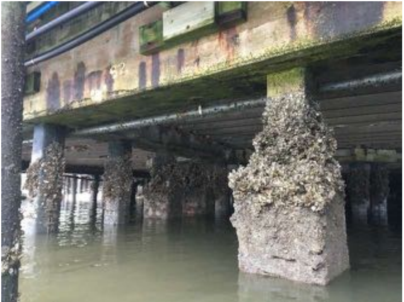
1.12~ West side of substructure looking northeast. Concrete beams with multiple horizontal cracks in bottom and side faces. Marine growth on piles.
