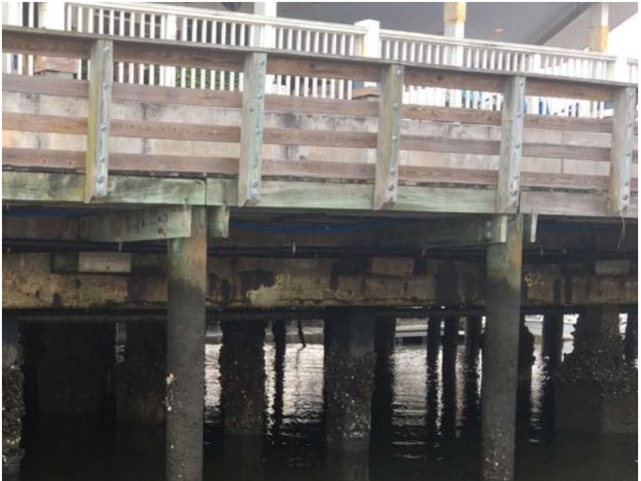
1.04~ Enlarged View of West Elevation looking at the center of the building exterior. Reinforced concrete beam / pile cap marked "B1" & "B2" by others in previous condition assessment with horizontal cracking at bottom of beam.
