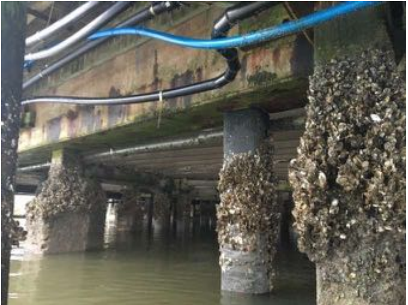
1.10~ Western portion of substructure looking northeast. Lower double tees with missing portions of their stems. Concrete beams with horizontal cracking and spalled concrete. Piles with marine growth.
