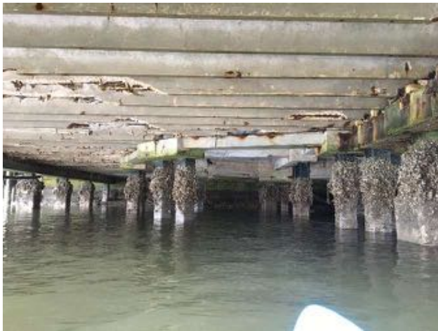
1.28~Northern portion of substructure; Lower double tees with missing sections of the stem at points of bearing and along the span; Octagonal area beams in good condition; beam on righthand side of picture has horizontal crack near bottom; piles with marine growth.
