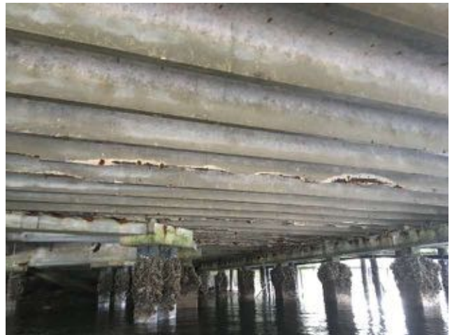
1.25~Lower double tees with missing sections of the stem along the span; concrete beams in fair condition; piles with marine growth.
