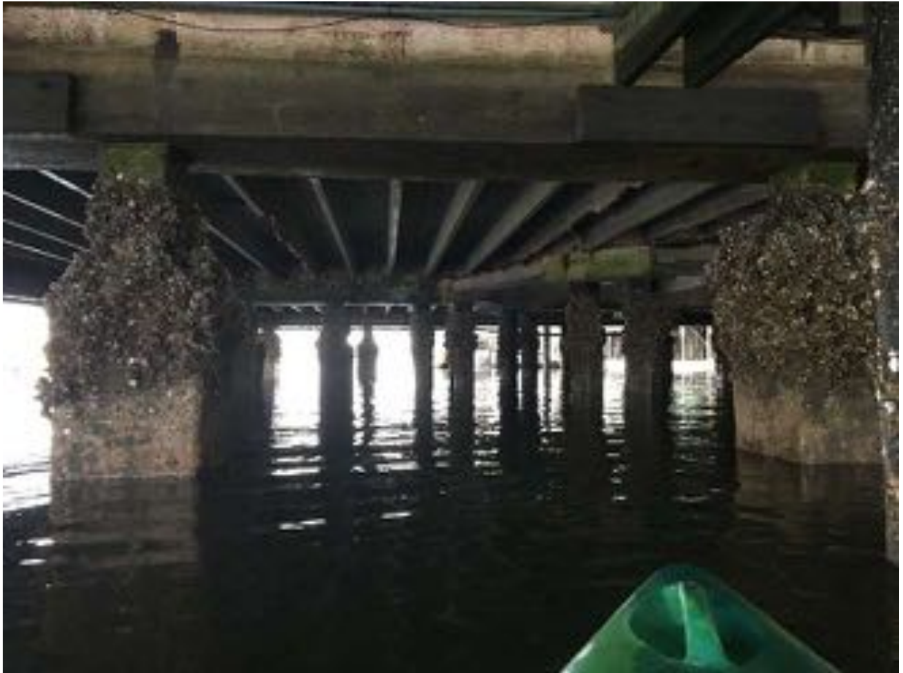
1.08~ South-central portion of substructure looking north. Lower double tees with missing portions of their stems. Concrete beams without visible defects. Piles with marine growth.
