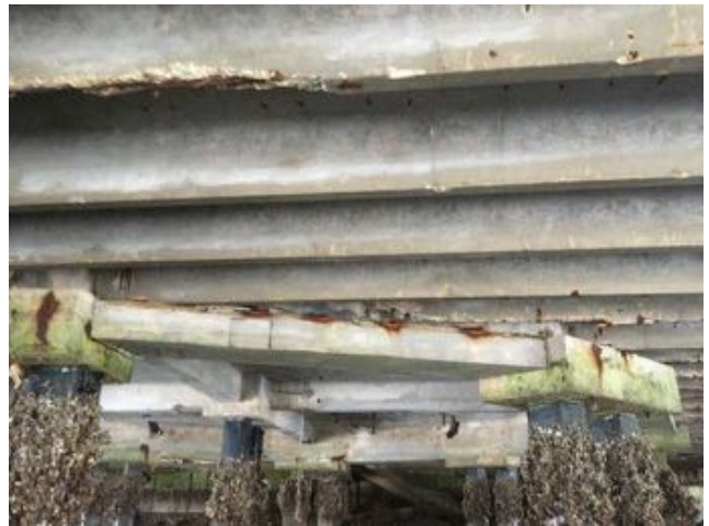
1.27~Lower double tees with missing sections of the stem along the span; concrete beams in good condition; piles with marine growth.
