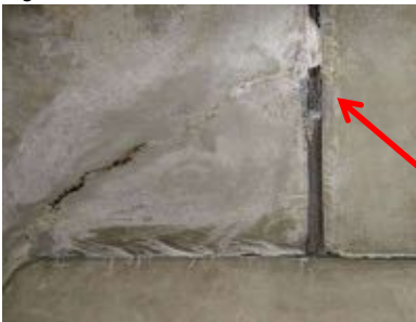
Figure 8: Leaking and Leaching Concrete
