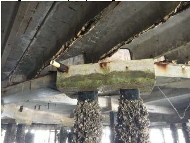
1.20~ Lower double tees missing stems. Concrete beam in Octagon area with patching and surface.
