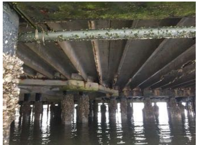
1.31~ Northeast area of substructure looking south; Lower double tees missing sections of the stem at points of bearing and along the spans; Octagonal area beams in fair condition with some patching; beam in picture foreground has cracking and spalling along bottom; piles with marine growth.
