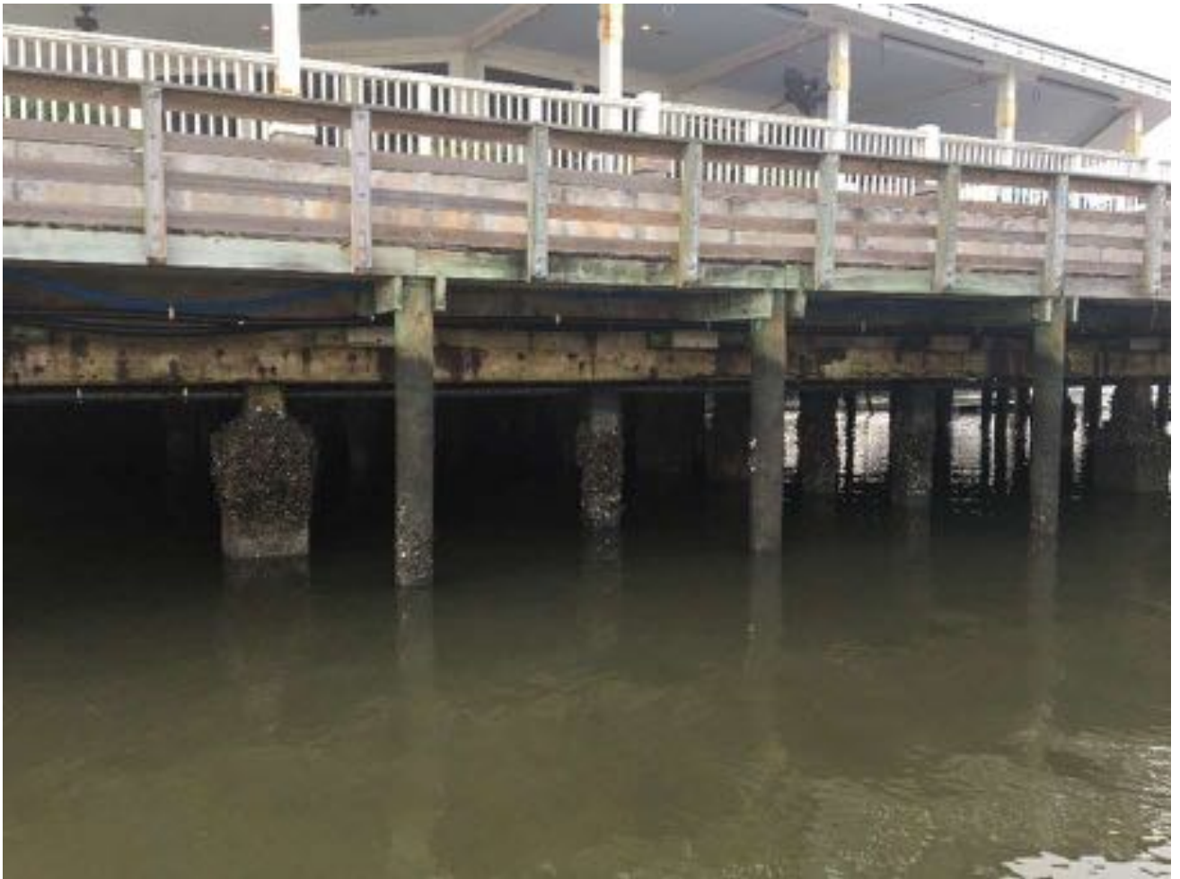
1.03~ West Elevation looking at the center of the building exterior. Concrete beams with multiple horizontal cracks. Marine growth on piles.
