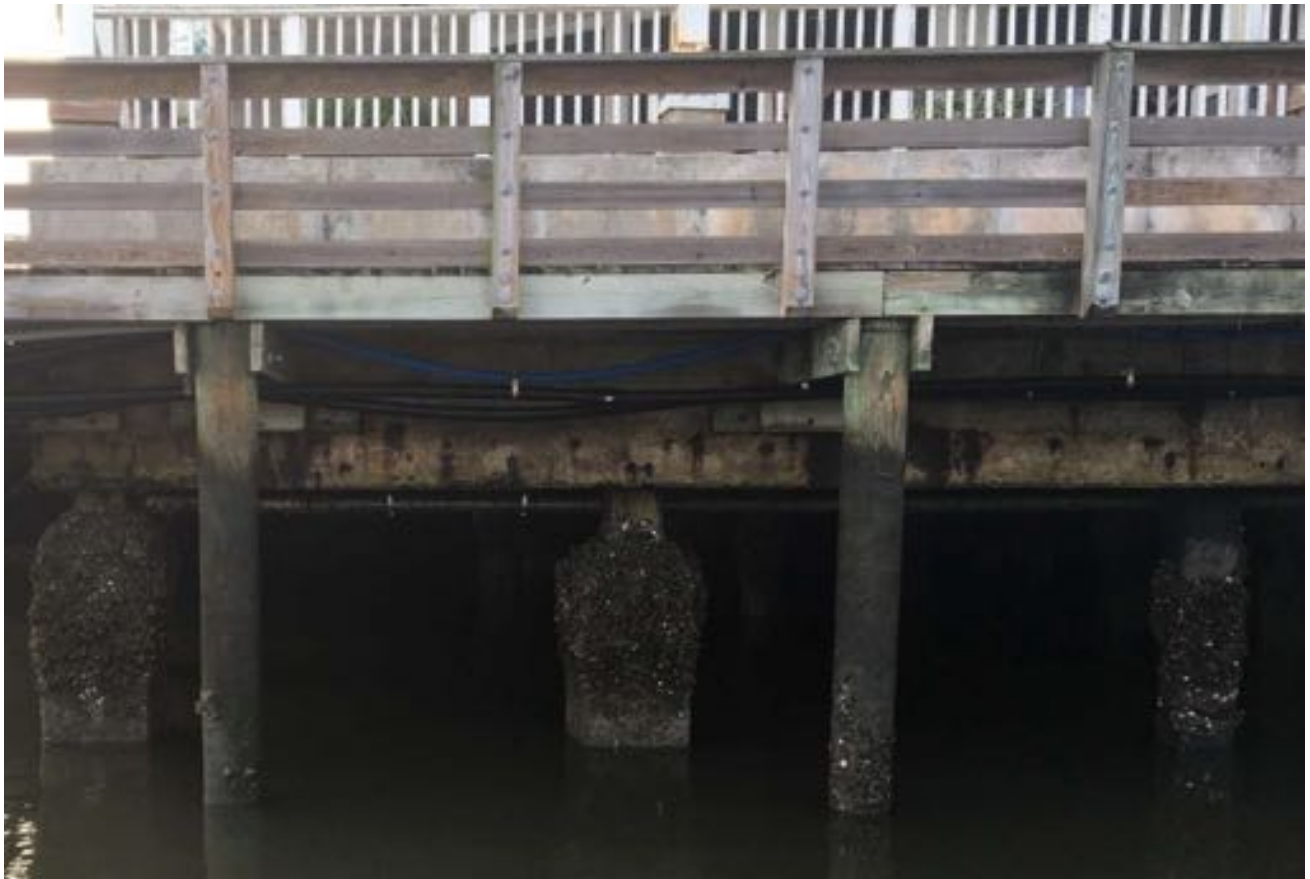
1.02~Enlarged view of West Elevation at the Northwest corner of the building. Horizontal cracking in the concrete beams and marine growth on piles.
