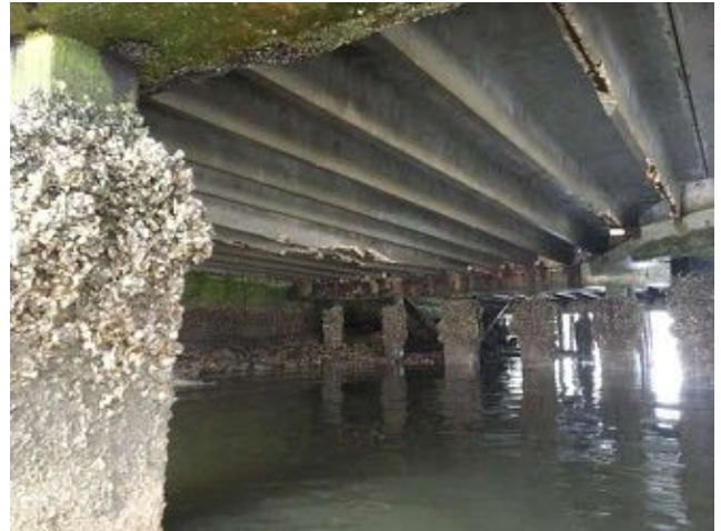
1.33~ Northeast area of substructure looking south; Lower double tees missing sections of the stem at points of bearing and along the spans; Octagonal area beams in fair condition with some patching; beam in picture foreground has cracking and spalling along bottom; piles with marine growth.
