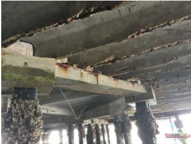
1.19~Lower double tees missing stems. Concrete beam in Octagon area with prior patching.
